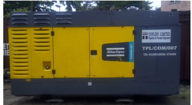
ATLAS COPCO AIR COMPRESSOR
