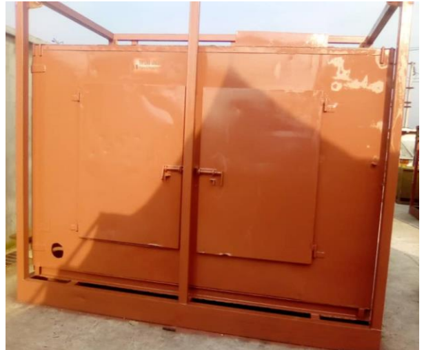
150KVA PERKINS 1006TAG DIESEL GENERATOR
